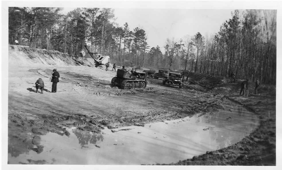
CCC constructing fish rearing pools. (photo courtesy of National Archives, Atlanta, Georgia)
